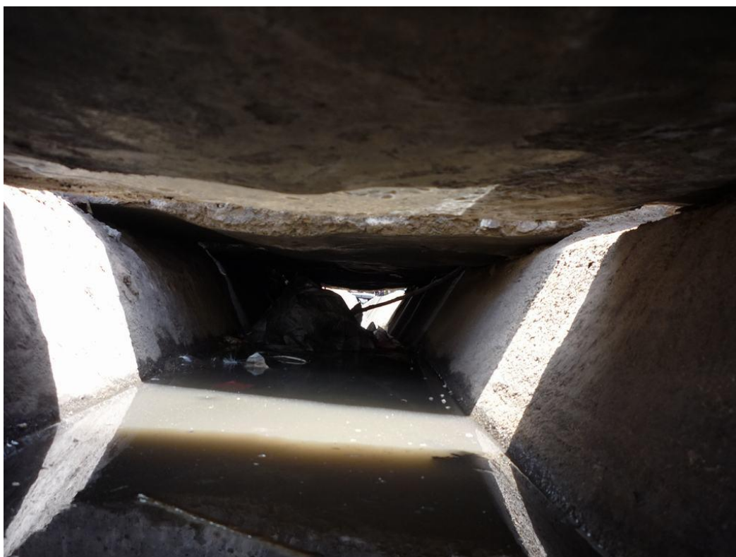
Figure 3-49: Secondary channel in Bairro Mafalala. Blocked underneath the concrete slabs which were placed on top of the channel for pedestrian crossing
