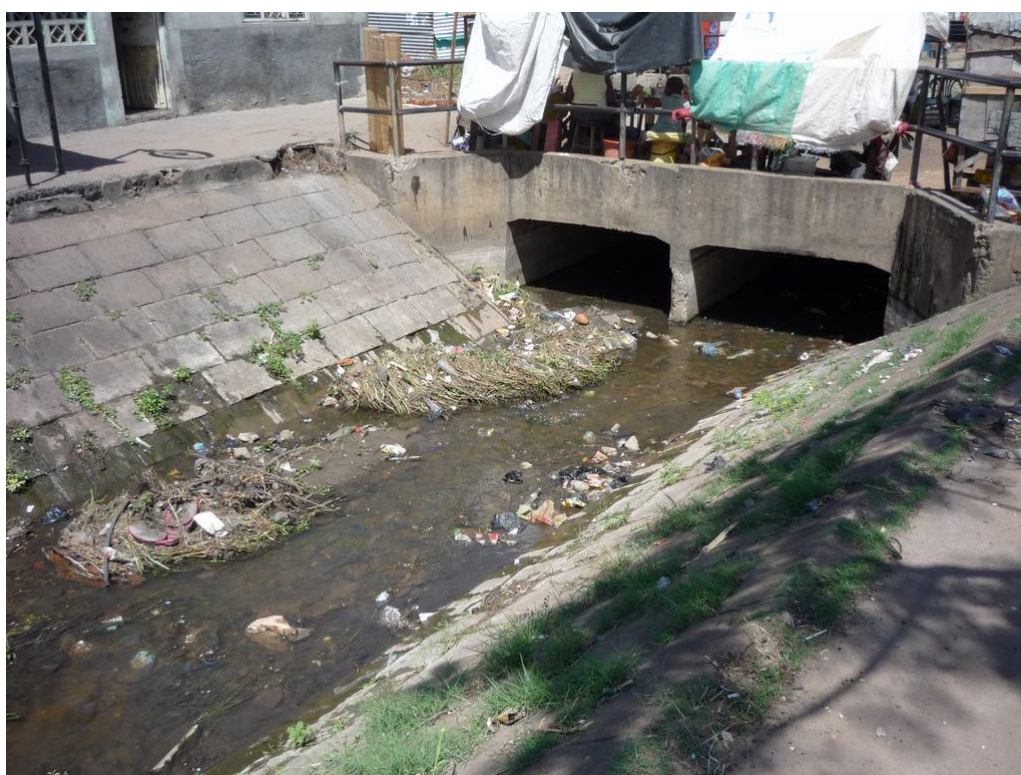
Figure 3-36: Main storm water channel along the Av. Acordos de Lusaka in Bairro Maxaquene A with a "base flow" of approx. 10 l/s household wastewater and with solid waste deposits.
