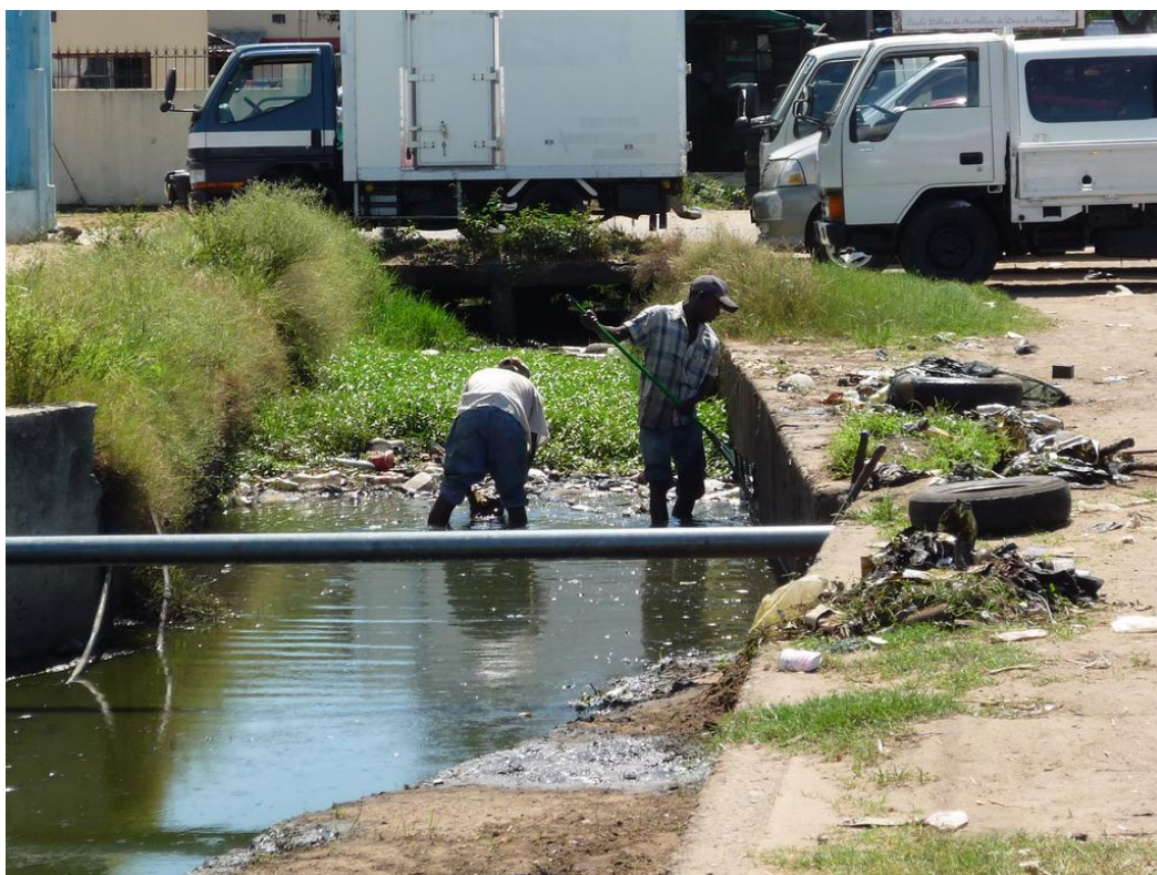
Figure 3-53: Same as above. The workers who are cleaning the channel do not have suitable tools for successfully clearing the channel.
