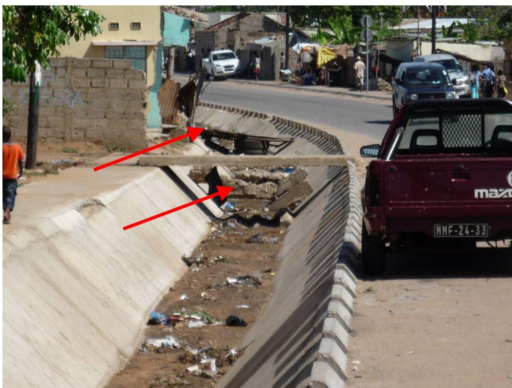
Figure 3-42: Secondary channel in Bairro Maxaquene: blocked intentionally by residents in order to get access to their houses
