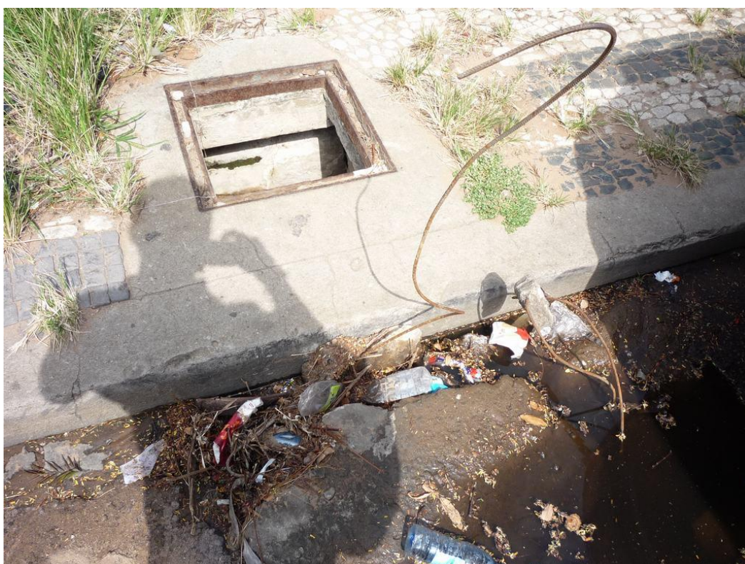
Figure 3-46: Storm water inlet in the cement city of Maputo: blocked by solid waste
