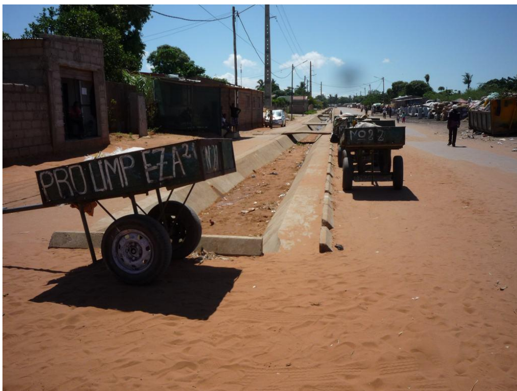
Figure 3-55: Secondary channel in Bairro Sommerschild, blocked with sediment.
