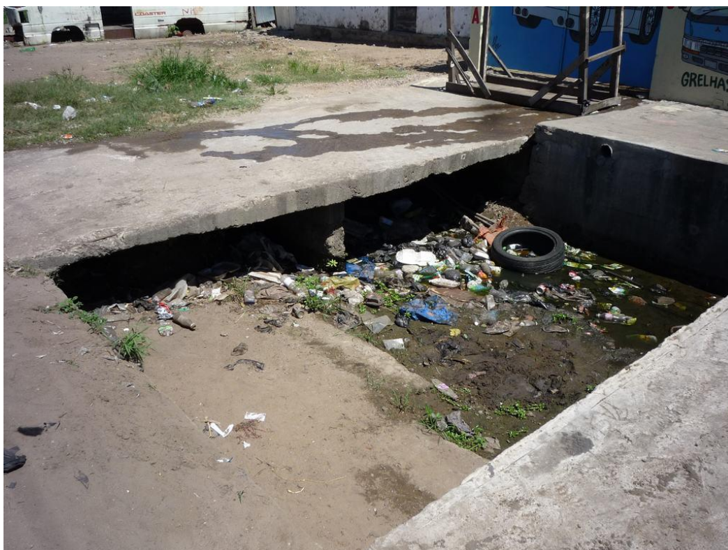
Figure 3-51: Secondary channel in Bairro Maxaquene. Almost completely blocked by solid waste
