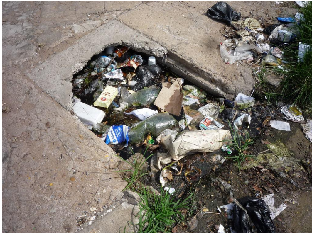
Figure 3-44: Storm water inlet in the cement city of Maputo: blocked by solid waste
