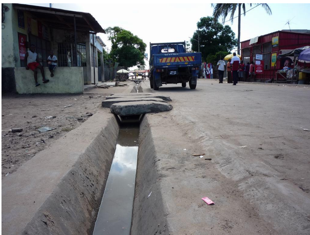
Figure 3-48: Secondary channel in Bairro Mafalala. Blocked underneath the concrete slabs which were placed on top of the channel for pedestrian crossing
