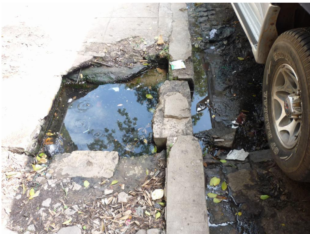
Figure 3-45: Storm water inlet in the cement city of Maputo: blocked, water cannot enter the sewer system
