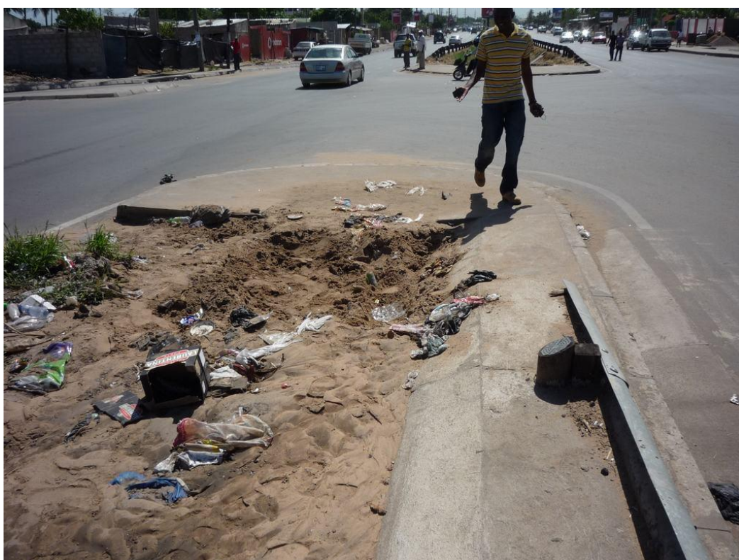
Figure 3-40: Upstream part of primary storm water channel in Av. Joaquim Chissano (downstream view), completely blocked with sediments
