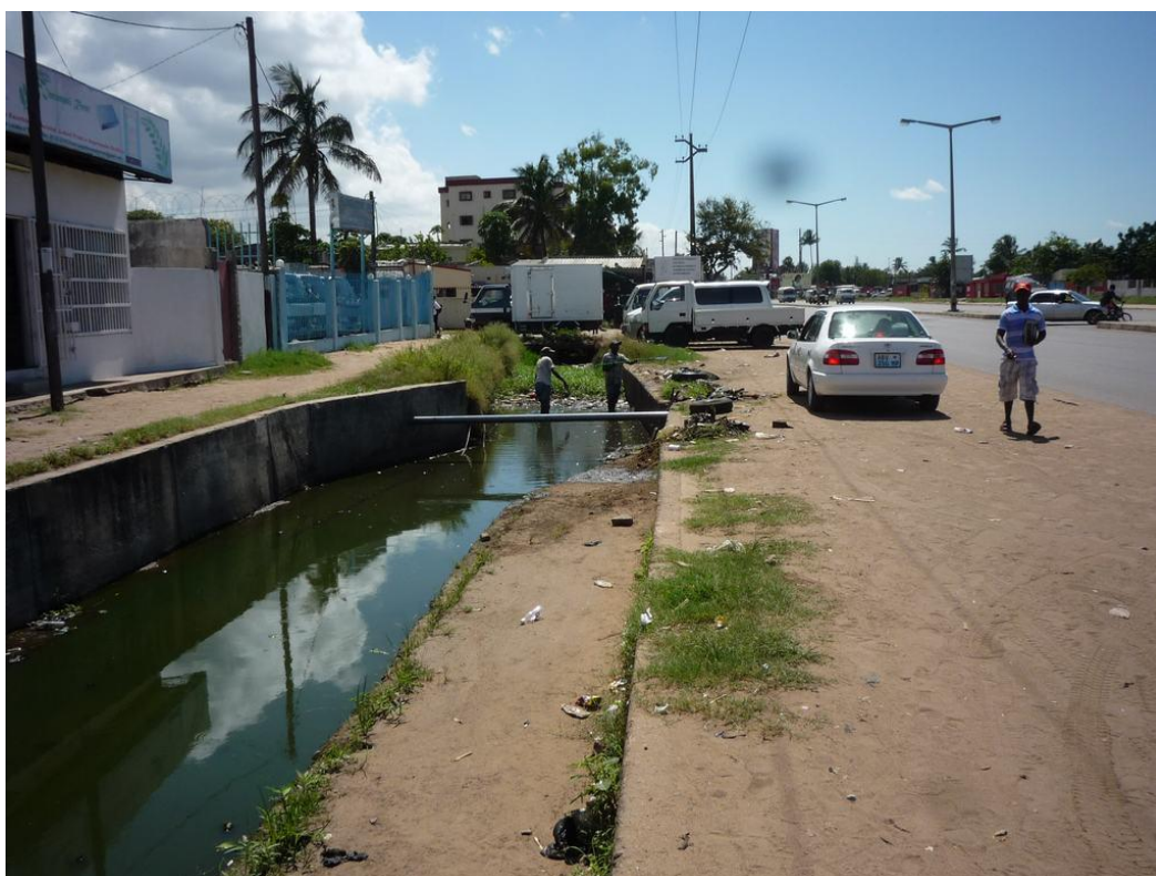
Figure 3-52: Drainage channel near Bairro Mafalala, blocked by solid waste and vegetation.
