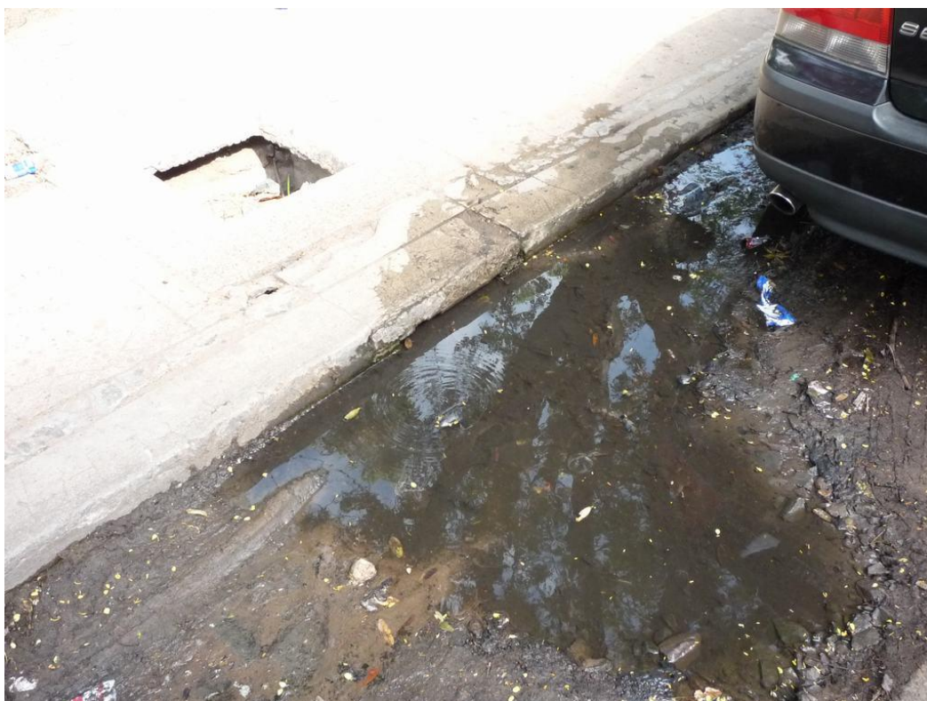
Figure 3-47: Storm water inlet in the cement city of Maputo: blocked, water cannot enter into the sewer system
