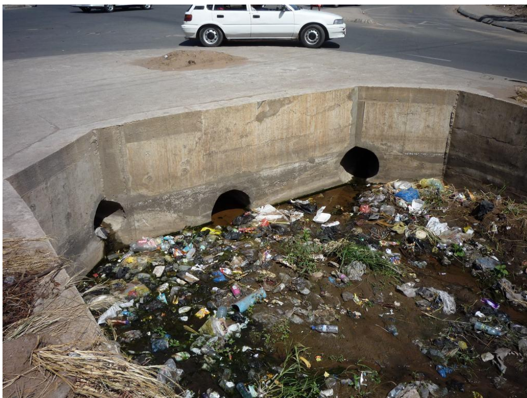
Figure 3-41: Inflow of several secondary channels into primary storm water channel in Av. Joaquim Chissano, directly downstream of blocked channel shown in Figure 3-39 and Figure 3-40
