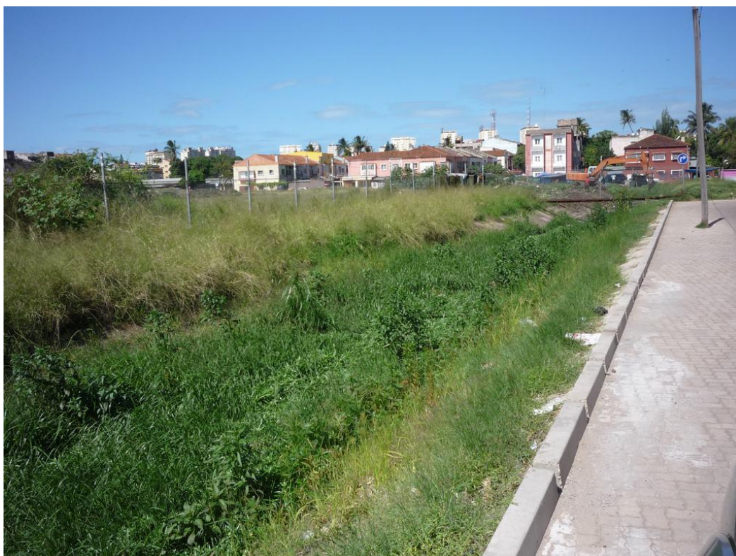
Figure 3-43: Storm water channel, completely blocked by vegetation
