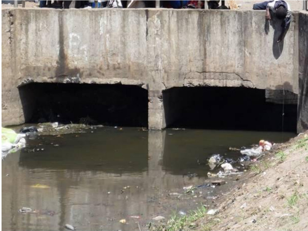
Figure 3-33: Culvert at the storm water channel along the Av. Acordos de Lusaka in Bairro Maxaquene A
