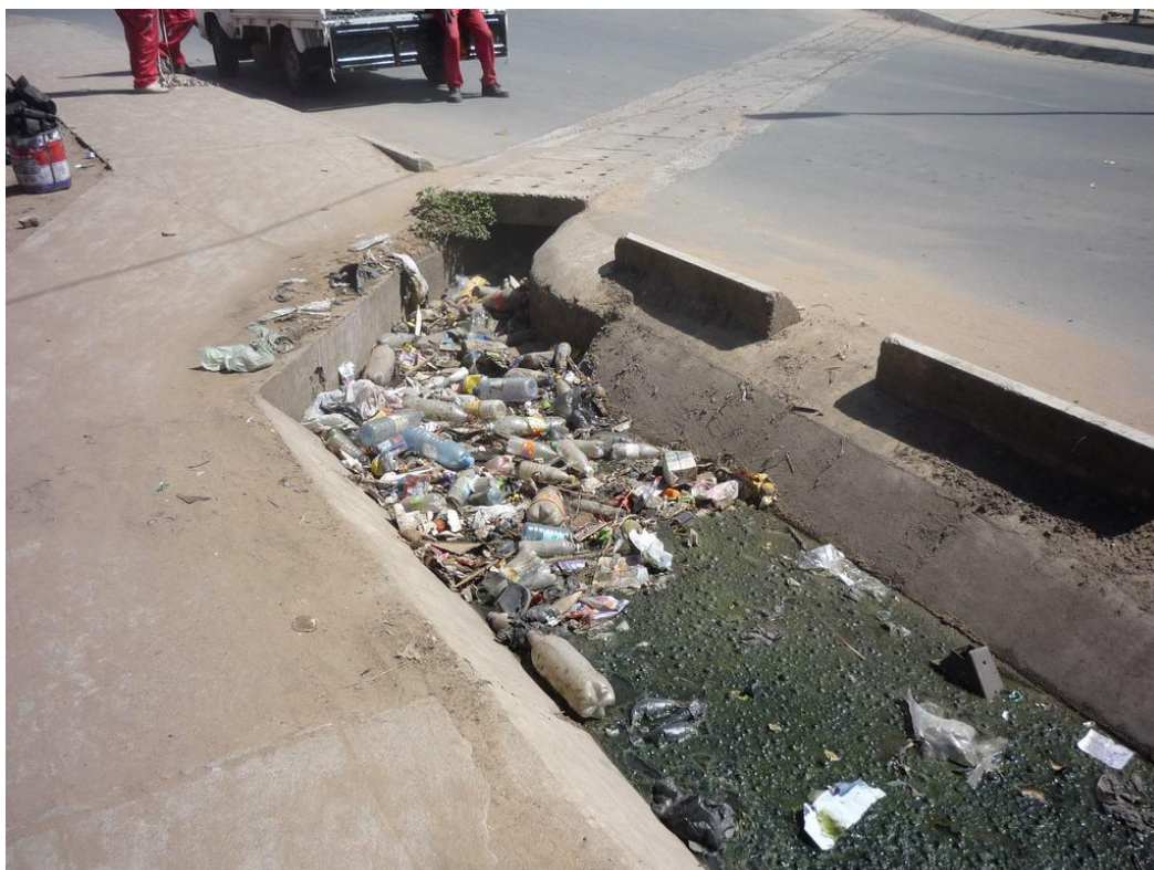
Figure 3-38: Secondary channel in Bairro Maxaquene A, out of operation due to blockage by solid waste
