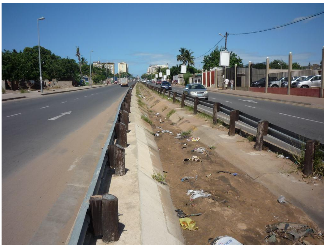
Figure 3-39: Upstream part of primary storm water channel in Av. Joaquim Chissano (upstream view), completely blocked with sediments
