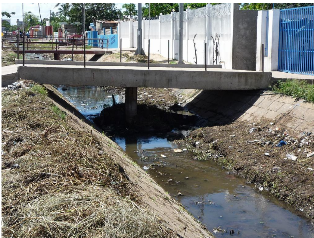
Figure 3-37: Bridge over the storm water channel along the Av. Acordos de Lusaka which is acting like a partly blocked culvert due to deposits of bulky solid waste
